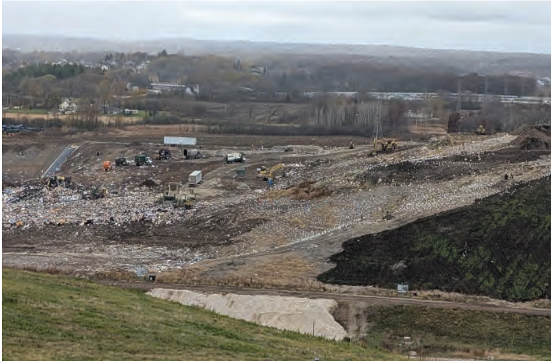
Southeast corner of Phase 3 being brought up to cresting grade, cover being placed as slopes are reached
